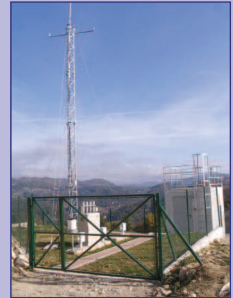
Desinic Air Quality Monitoring Station
